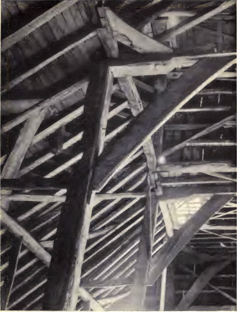
THE CRACKED BEAM OF THE SHIP
